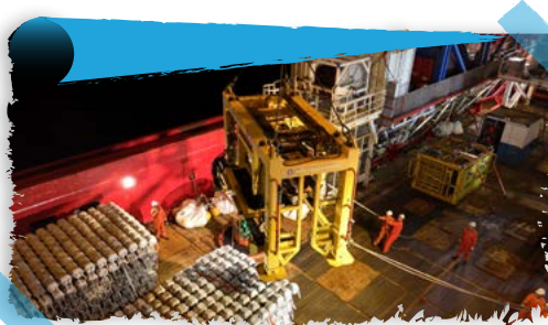
China's First Deepwater Submarine Pipeline Leak Plugging Practical Offshore Drill in Progress
