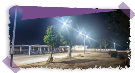
Newly Installed Street Lamp
